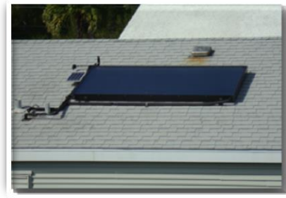
A solar water heating panel installed on a home in Big Pine Key.
