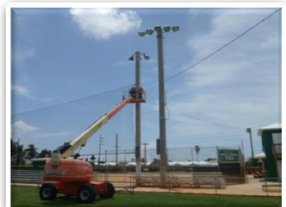
Key West ball field lighting retrofit
