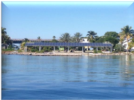
Pigeon Key solar panels
