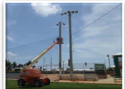
Key West ball field lighting retrofit
