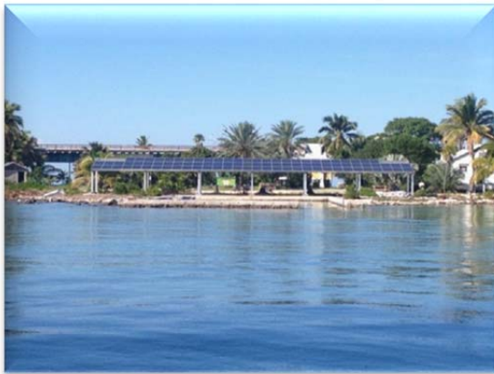
Pigeon Key solar panels
